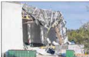
Severe damage is seen to the corner of the ImOn Ice Arena in Cedar Rapids on Tuesday. (Andy Aheya photo/The Gazette)
