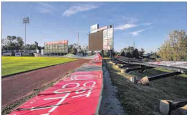
The back wall of the outfield at Veterans Memorial Stadium is seen collapsed Tuesday in Cedar Rapids. (Andy Aheya photo/The Gazette)
